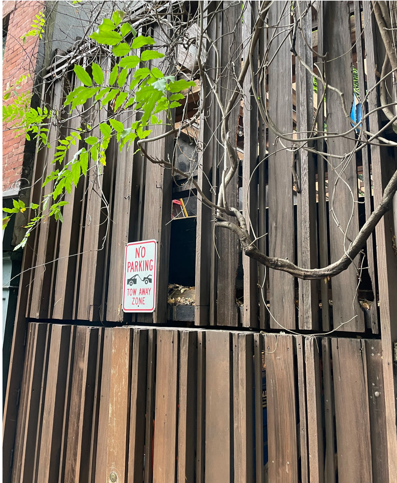
View from State Street - 2023 Fence Condition
