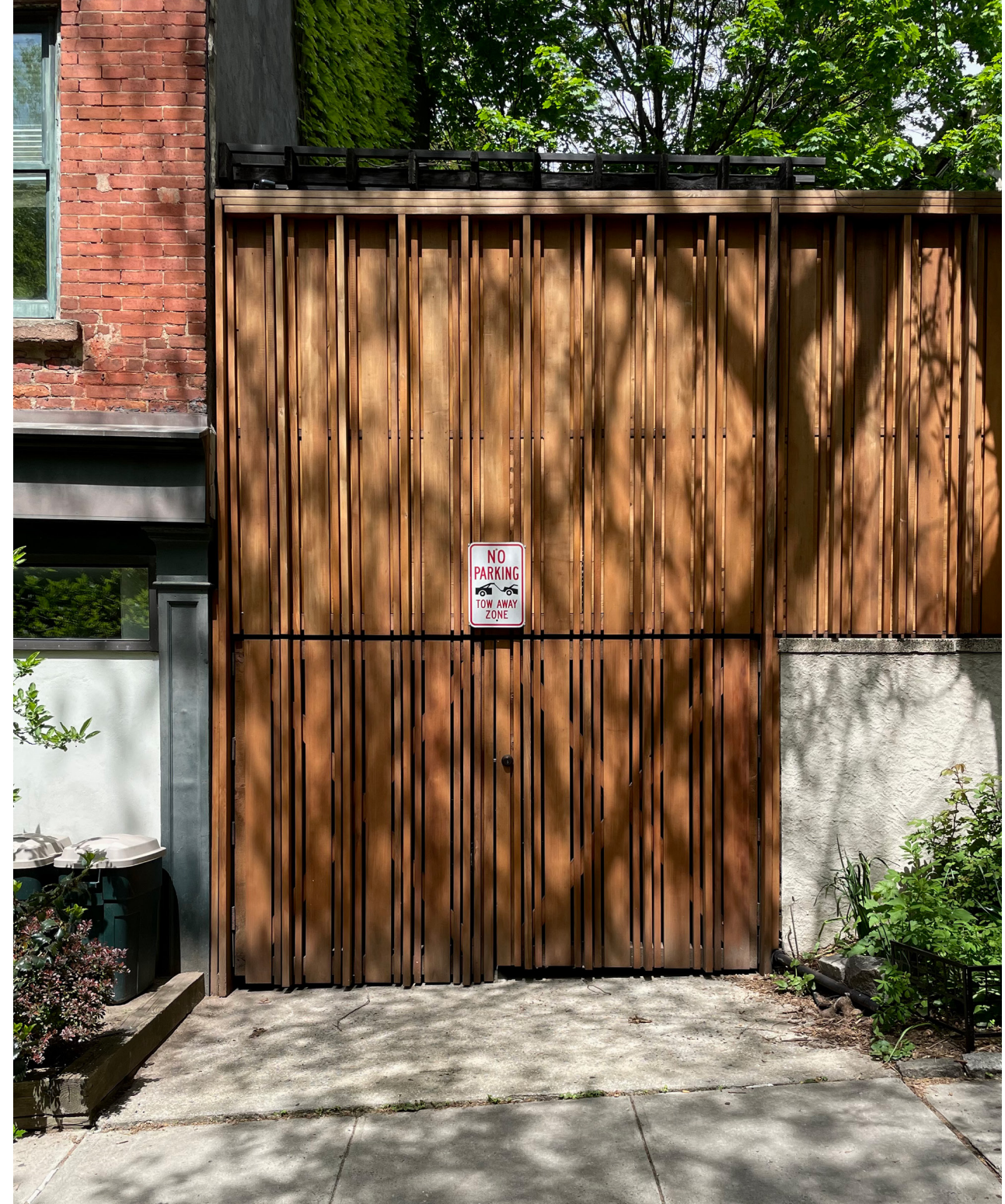
View from State Street - 2024 Fence Condition
