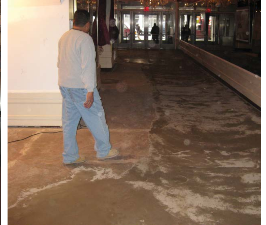
VIEW C - REMNANTS OF EXISTING LOBBY TERRAZZO FLOORING UNDER CARPET IN POOR CONDITIONS, DAMAGED AND PATCHED
