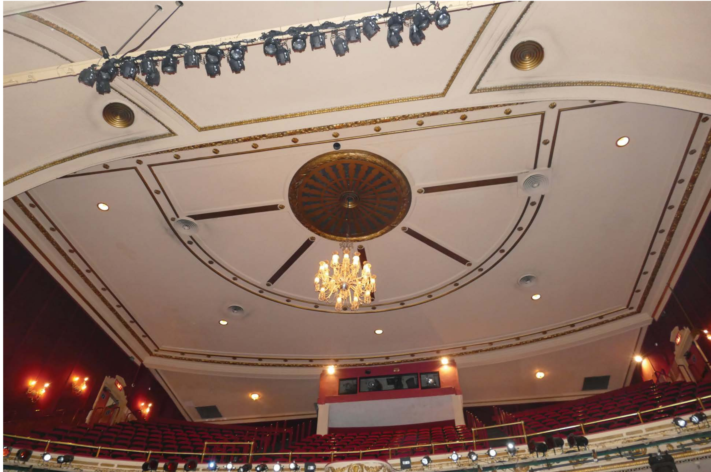
EXISTING AUDITORIUM CEILING CONDITIONS
