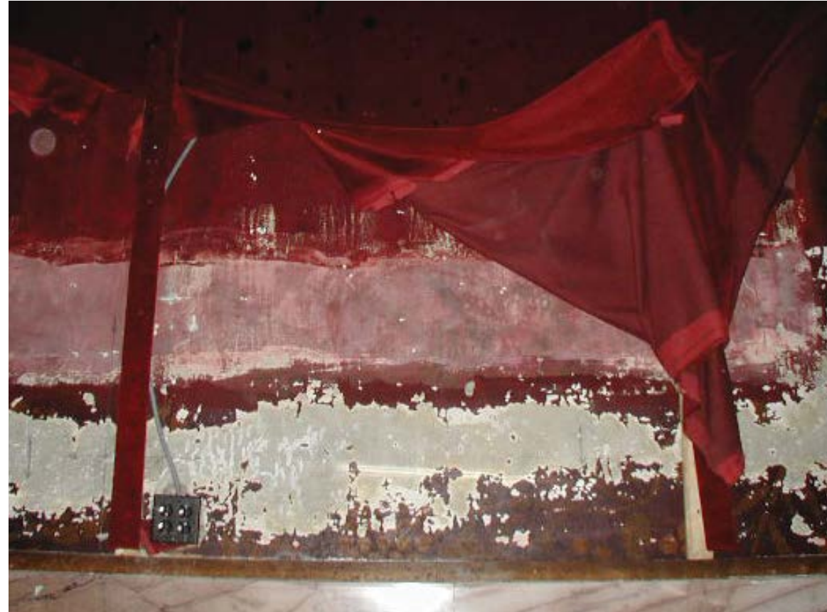
EXISTING PLASTER WALL CONDITIONS BEHIND FABRIC WRAPPED WALL PANELING
