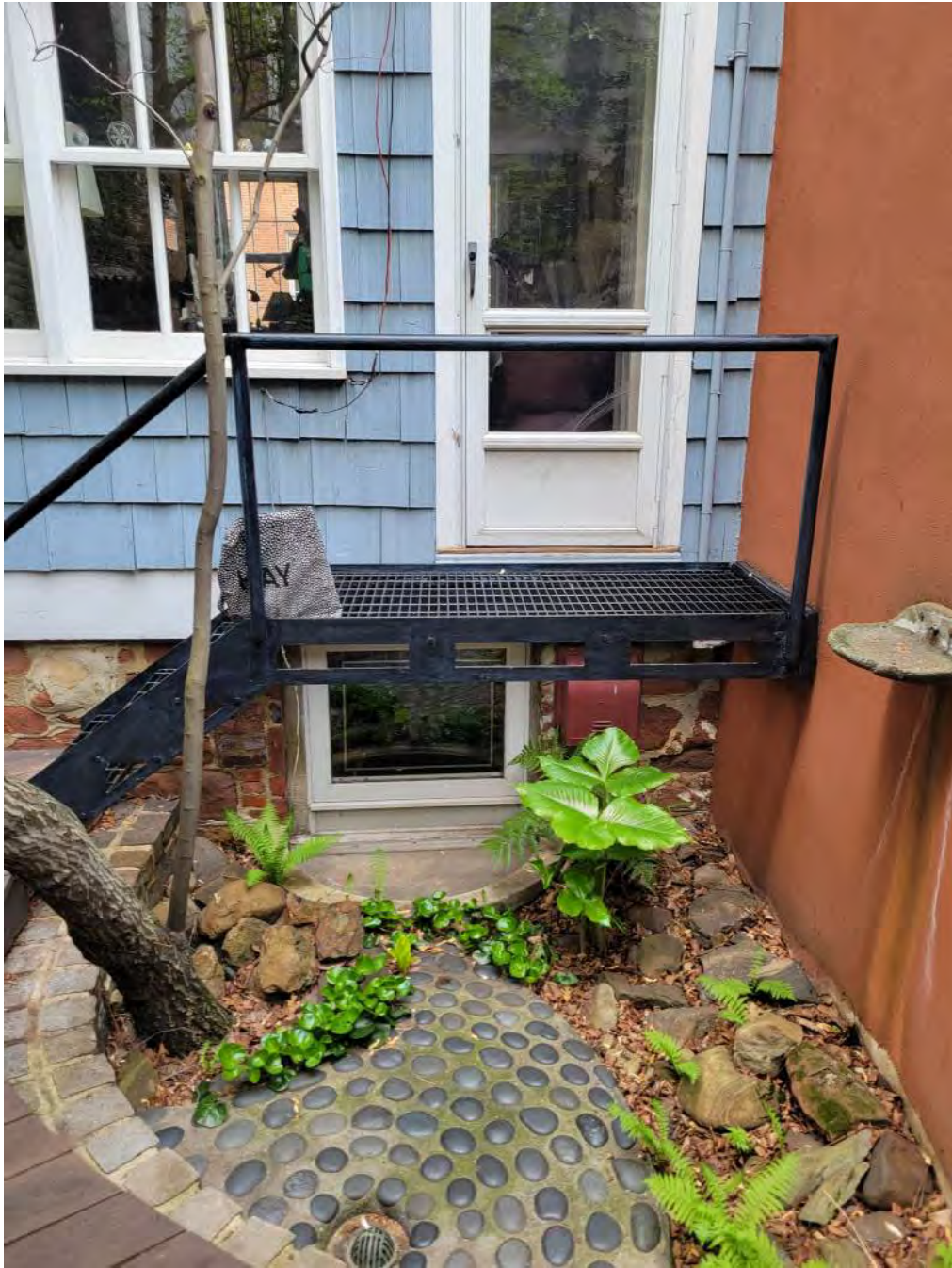
Existing Cellar Window
