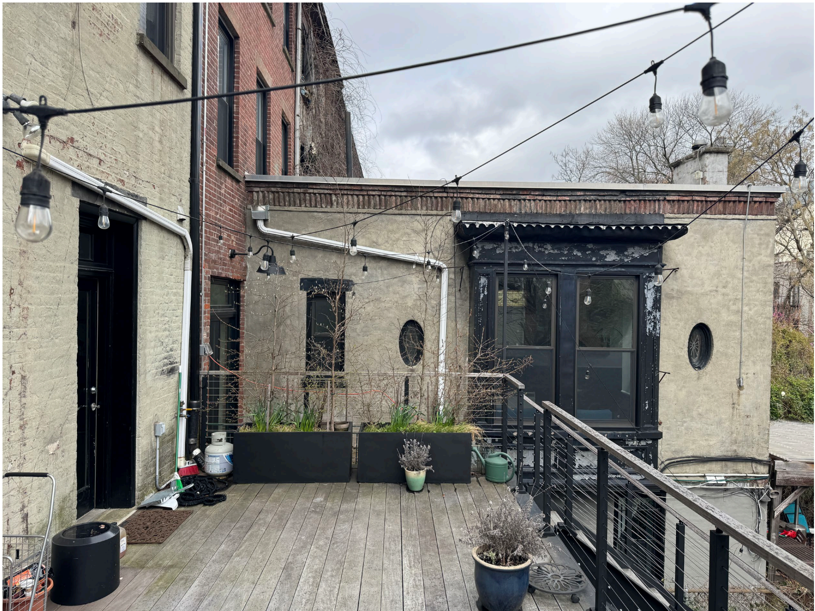
VIEW OF EXISTING 2-STORY REAR ADDITION OF 119 ST MARKS AVE – APPX 26 FT DEEP
