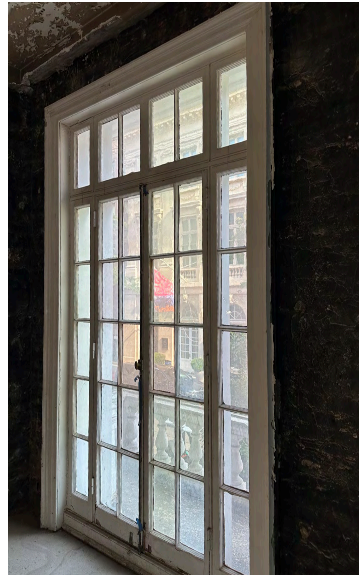
INTERIOR BALCONY DOOR CONDITIONS
