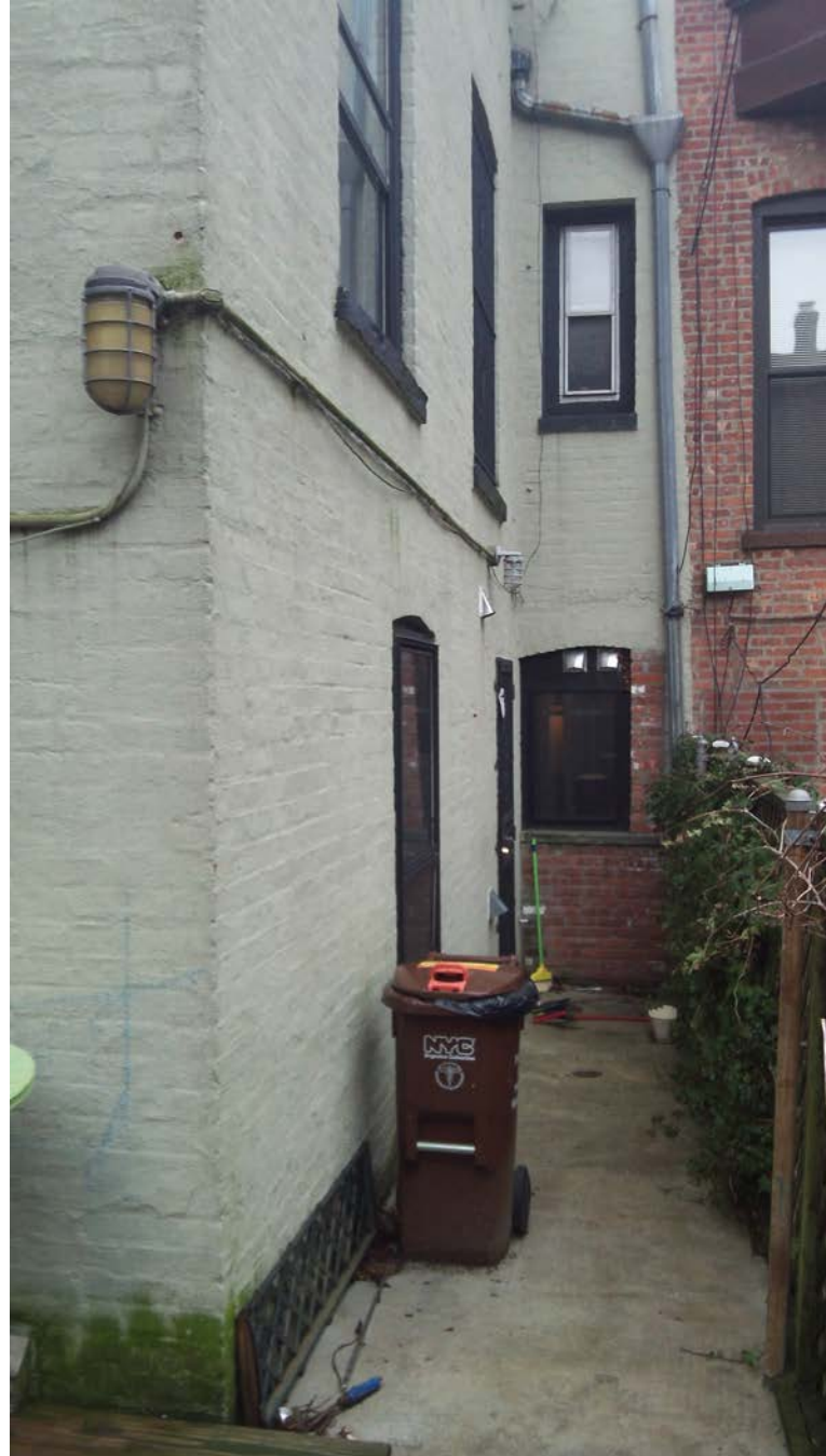
EX'G CONDITIONS AT WEST REAR FACADE
