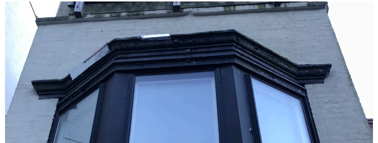
EX'G CONDITIONS AT TOP BAY WINDOW
