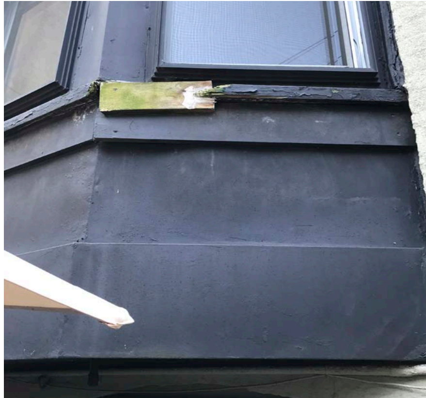
EX'G CONDITIONS AT BAY WINDOW LEFT SIDE
