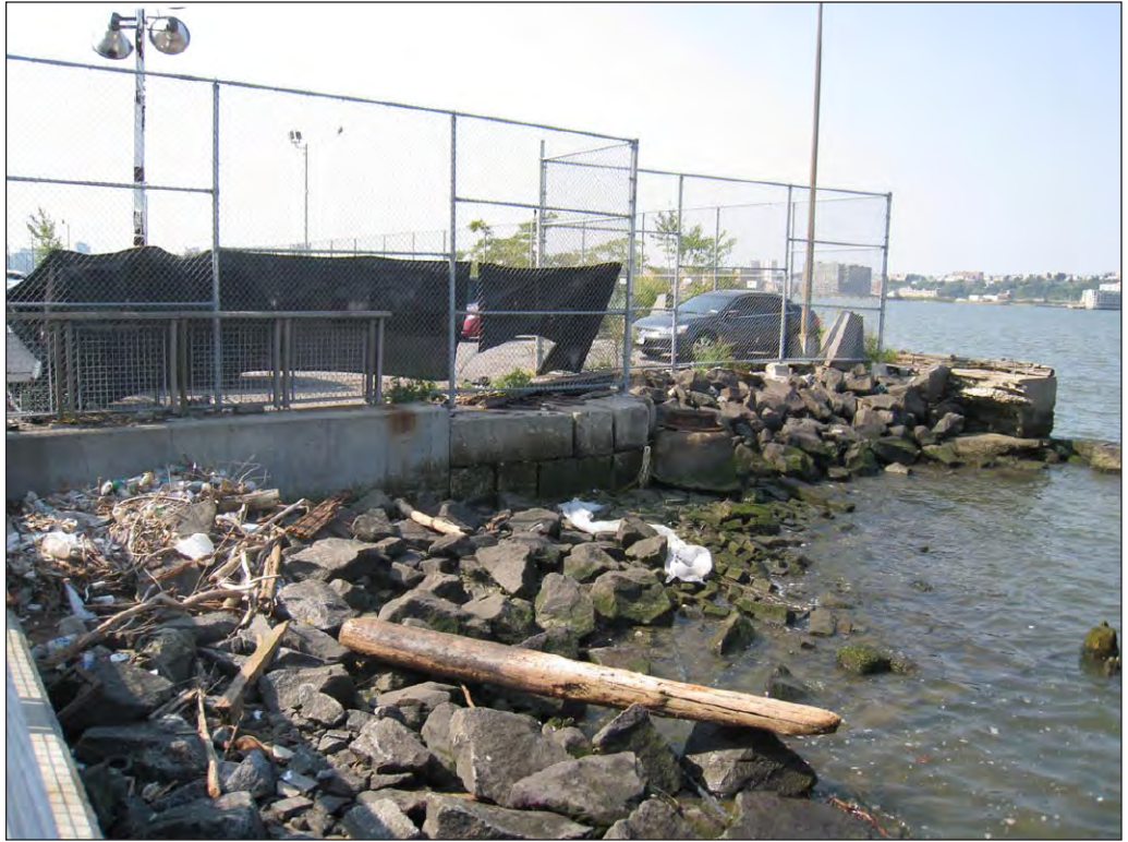
View of riprap and bulkhead on the Hudson River at West 34th Street 7
