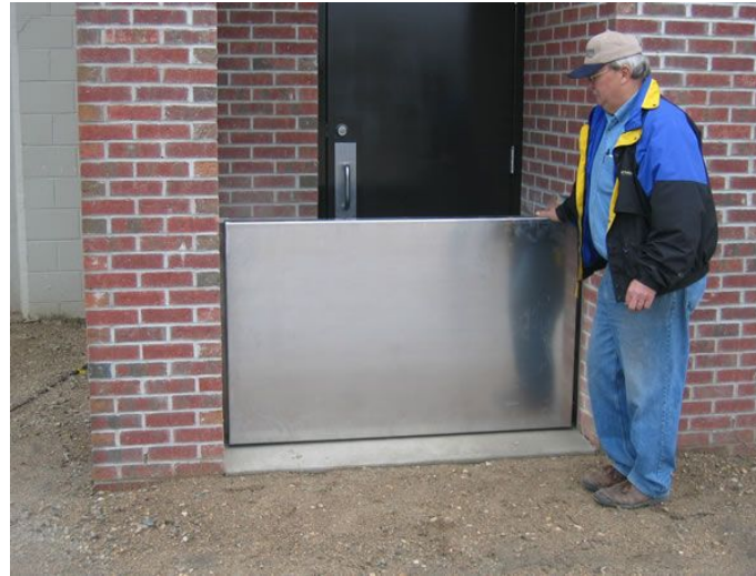
Deployable floodgate (currently allowed only at doors and operable windows)
