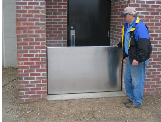
Deployable floodgate (currently allowed only at doors and operable windows)
