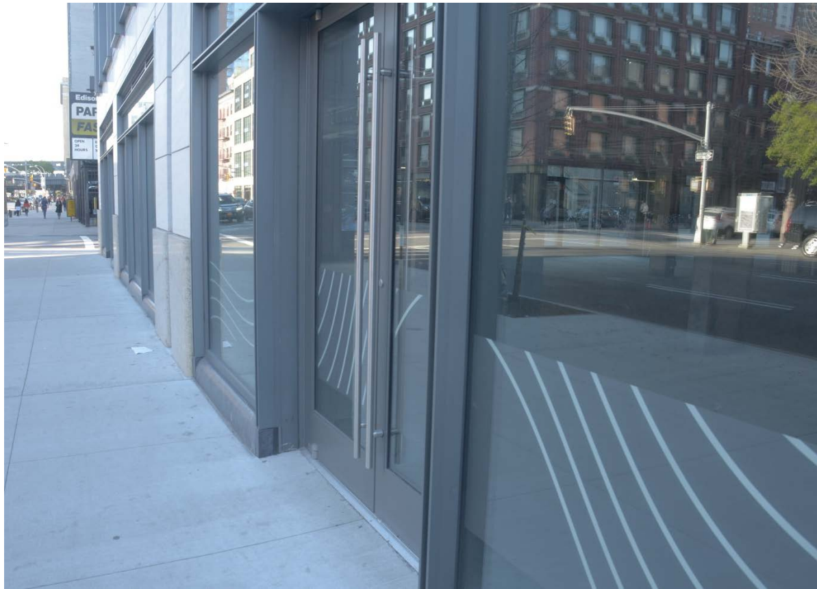
Commercial Ground Floor Existing Building with access at grade (deployable flood shields)
