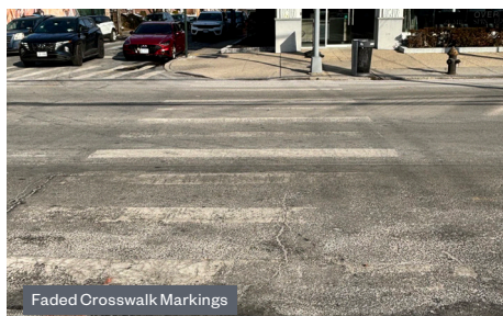
Faded Crosswalk Markings
