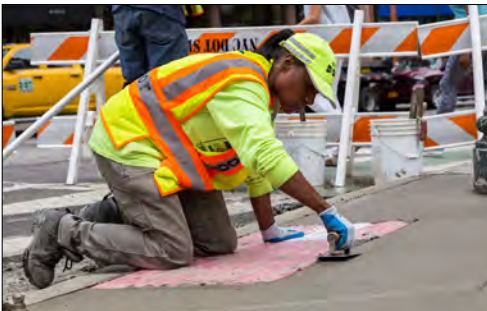
Above: A DOT employee installs a new pedestrian ramp. Right: A person in a wheelchair enters a sidewalk via a pedestrian ramp.
