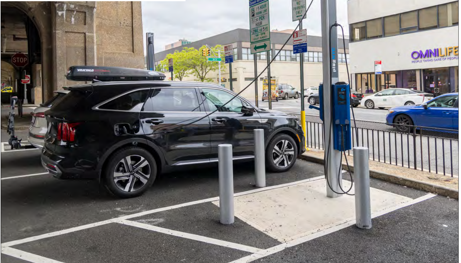
EV charging station at Queens Boulevard, Queens
